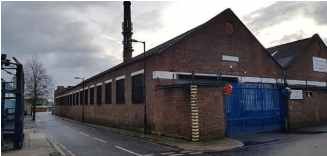
Figure 30: View of northern and western elevations and chimney of application site to be retained fronting Bianca Road.
